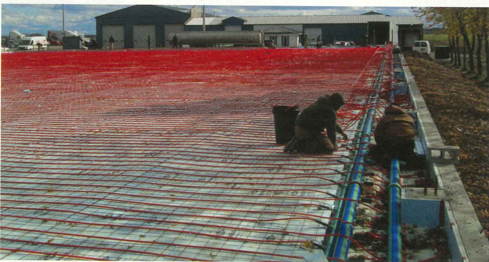
Armstrong Trucking is looking at adding another 25,000 sq ft of warehouse space this spring. This same system surely will be repeated thanks to its success.
